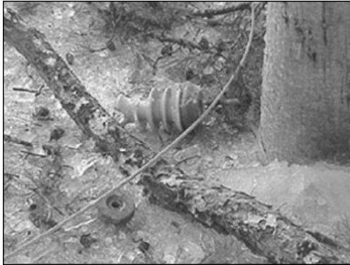
FIGURE 2-3: Little Rock, AR, December 29, 2000. Downed power cables are among the damage after a recent ice storm. (Photo by John Shea/FEMA News Photo.)
