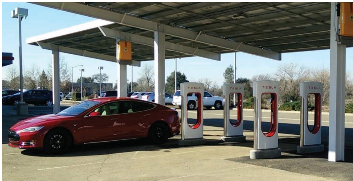
Figure 5. Tesla Supercharging Station
